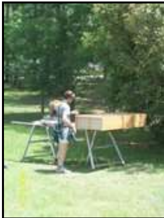
Above: Mukunda making wall shelves and reinforcing old bookshelves to support the weight of the books.
